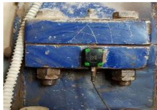
IOT sensor at Cooler Fan
